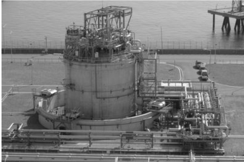
Figure 1: 1,000 m 3 Pilot LNG storage facilities
