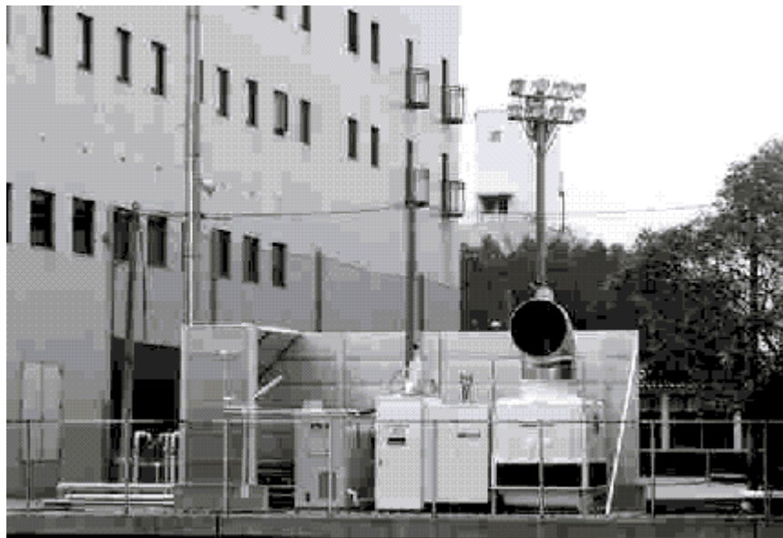
Photo2 TPC-50R with absorption chiller / heater installed Howa Sports Land
