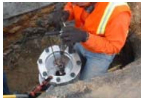
Figure 7: Pressure lock housing and manipulator being used to connect rod to conduit
