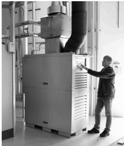
Figure 5 Capstone 30 kWe fitted with commercial version of high efficiency small-scale heat exchanger, developed by GET
