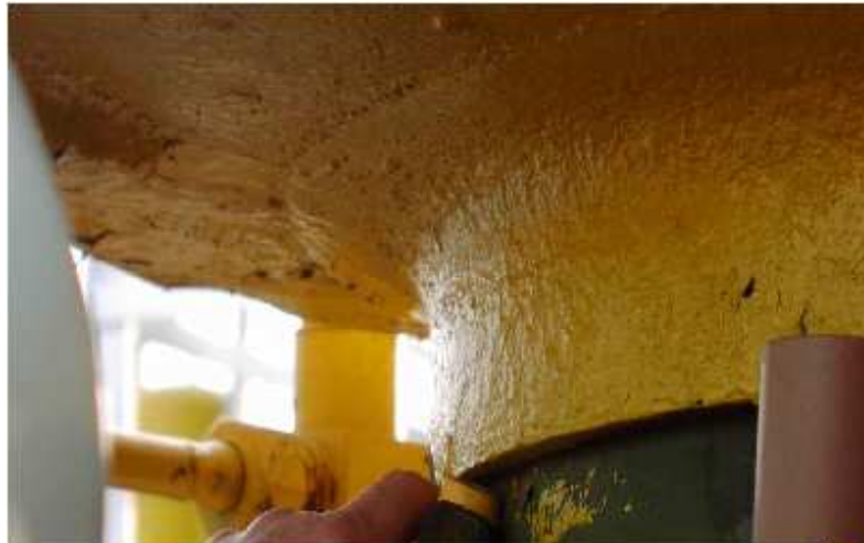
Screening of fittings at seperator
