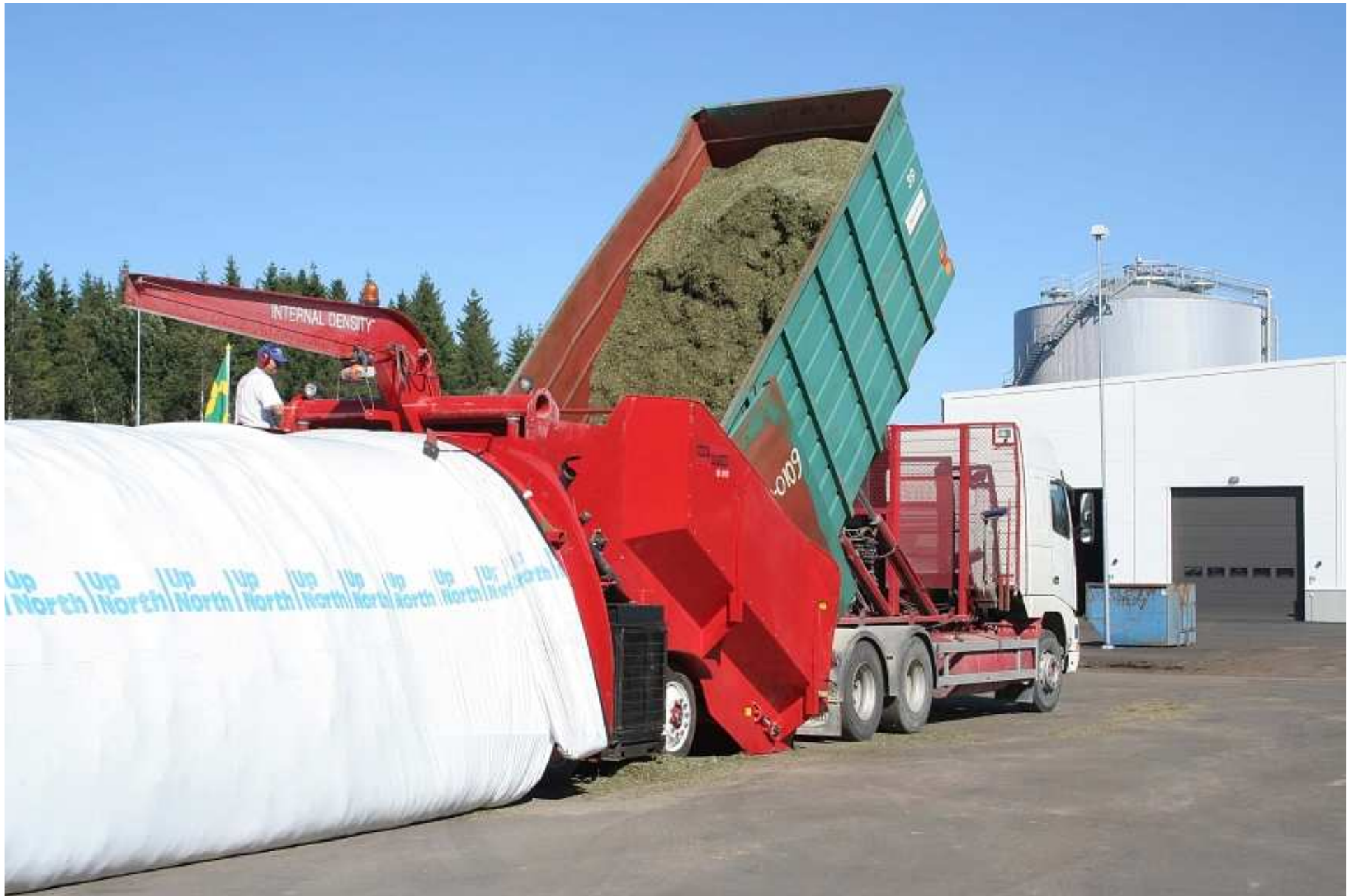
Västerås Biogas Plant, Sweden, Start up - 2005; Source: T. Al Seadi, Department of Bioenergy, SDU, Denmark
