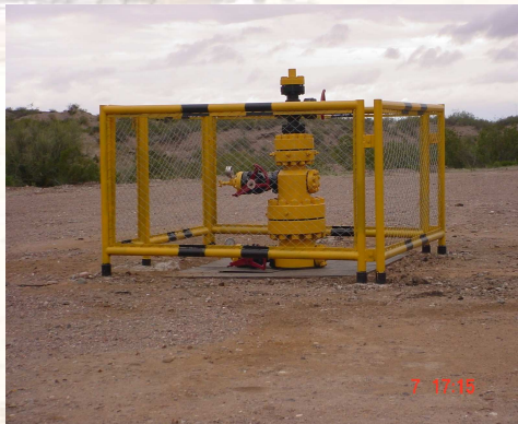
Gas monitoring well
