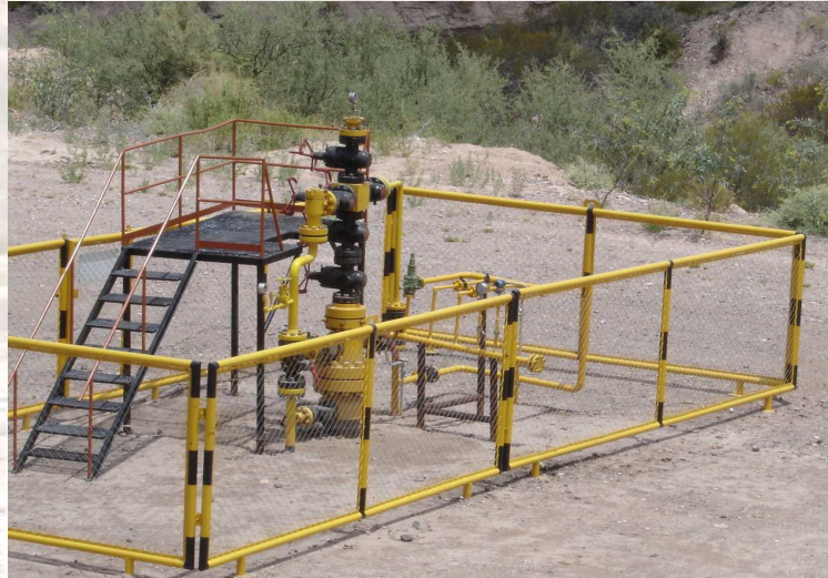
Injection / Withdrawal well
