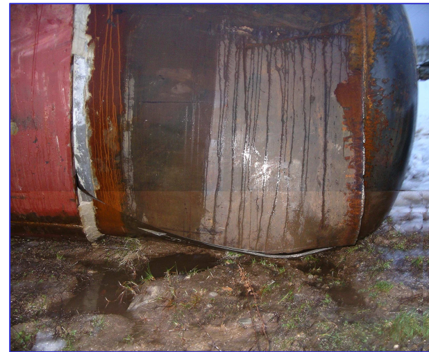
The sleeve fitting stopped longitudinal crack propagation. Further on the crack propagated crosswise along the sleeve fitting edge
