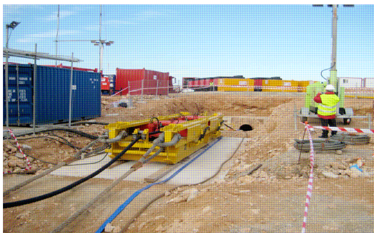
Figure 8.06 Ibiza Landfall Linear Winch
