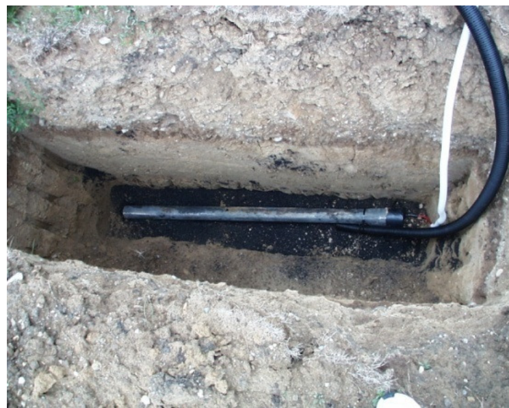
Figure 6 to 9: Photos from construction of active corrosion protection at the compressor station
