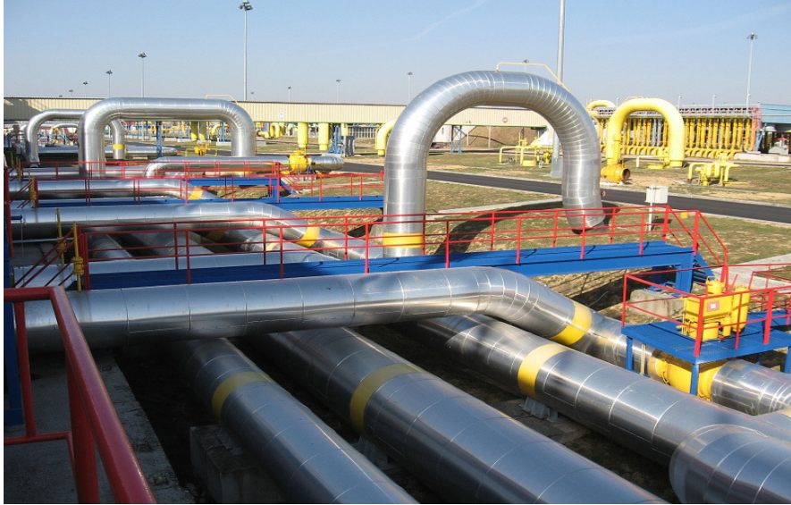
Figure 3. Pipeline systems at the compressor station
