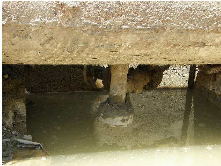
Figure No. 4. Decanting pipeline
