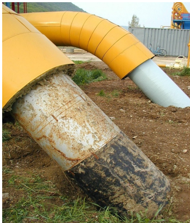
Figure 5. Original and repaired insulation at the point of ground-air passing
