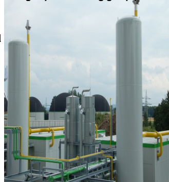
Biogas plant feeding gas pipeline
