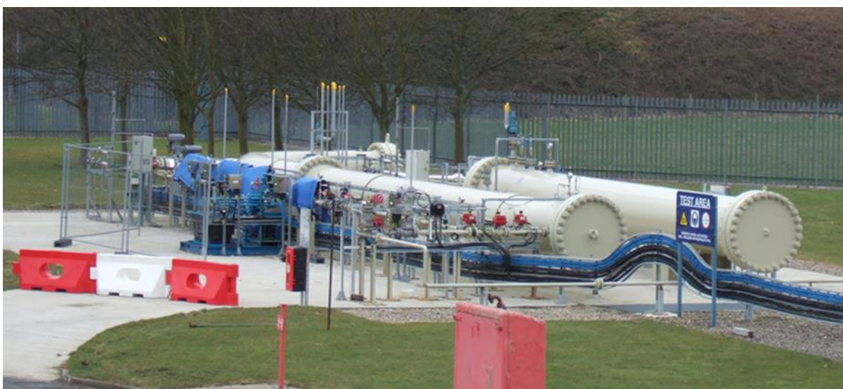
Figure 5: Photograph of the ANG field trial test facility
