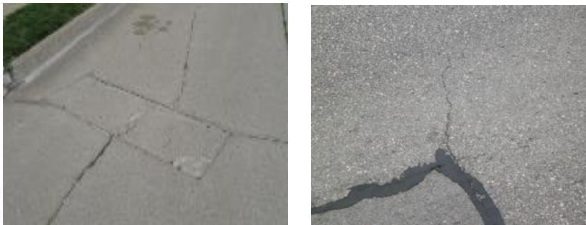
Figure 6. Pressure cracks emanating from the corners of traditional utility cuts
