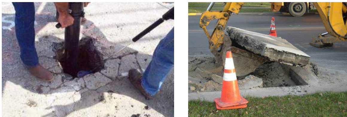
Figures 8 and 9. Damage around the utility cut caused by jackhammers and backhoes
