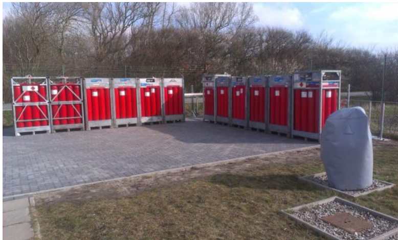
Fig. 1: Cylinder bundles installed at the pressure regulating station in Klanxbüll/Neukirchen for hydrogen injection into the distribution grid.
