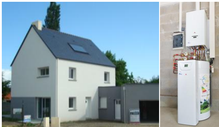
Figure 7: One of the field-test of an optimized solar thermal heater, with the monitoring system
