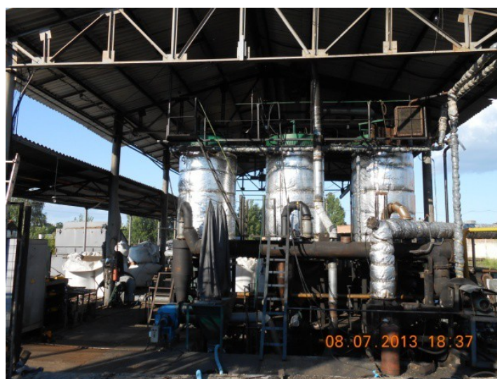
Fig.2. The plant for biomass gasification of 1,8 MW capacity
