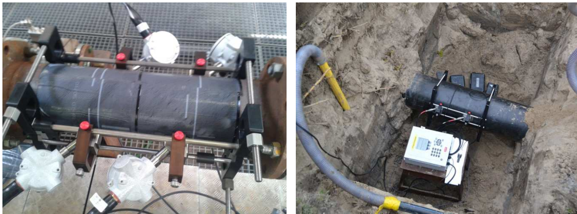
Figure 2 Clamp-on ultrasonic flow meters (left photo: built onto a pipe line in the test facility ; right photo: built onto one of the pipe line in the field)
