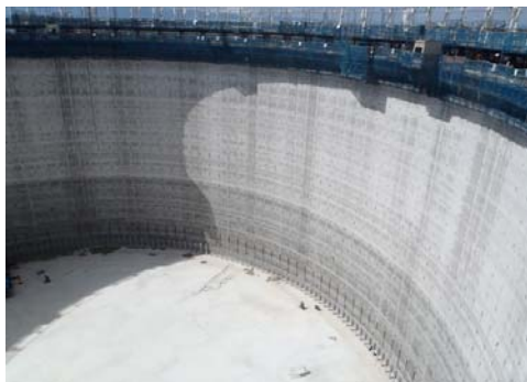
Picture 3. Inside of the outer tank
