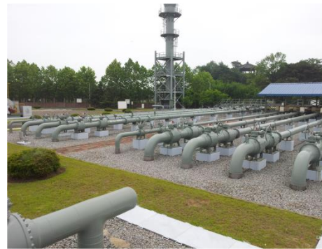
Fig. 1 The metering facilities of a gas station
