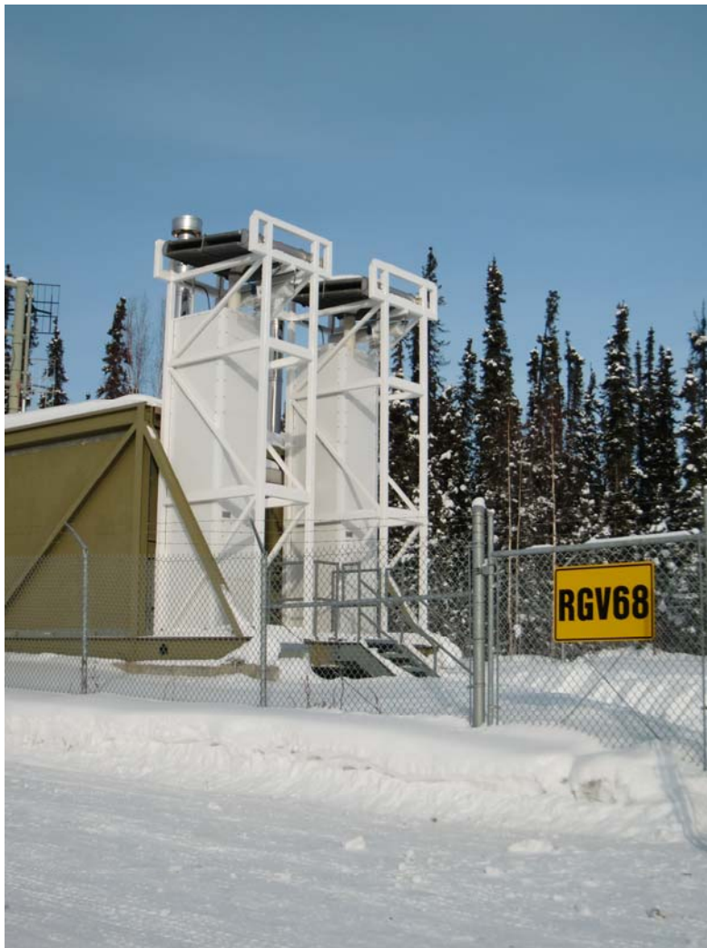
Figure 3: New 1200W CCVT units in existing RGV station
