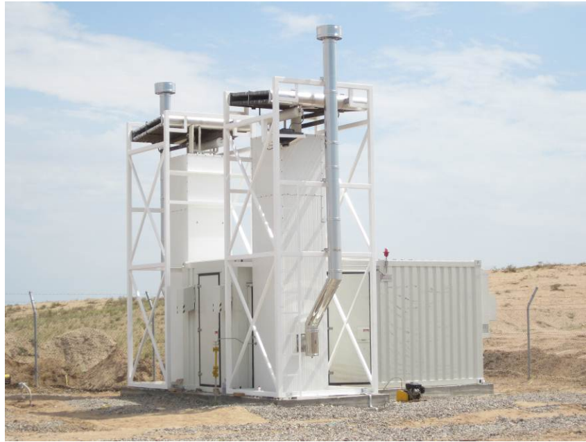
Figure 7: Energy Power System along Phase II of Kazakhstan – China gas pipeline
