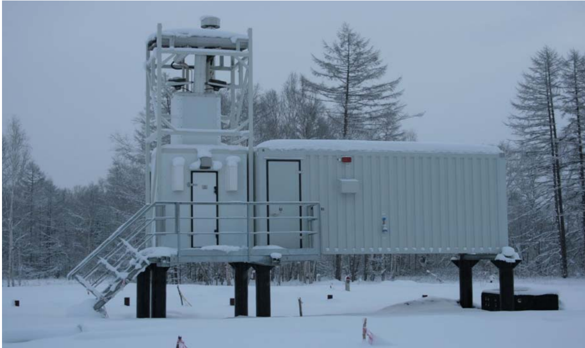
Figure 6: Energy Power System along Sakhalin II project
