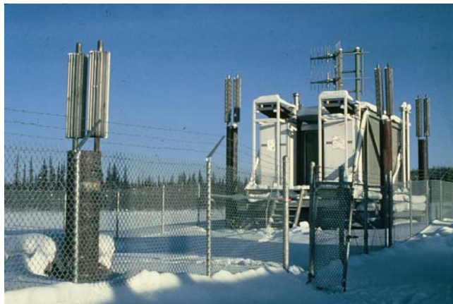
Figure 2: CCVTs on the Trans - Alaska Pipeline
