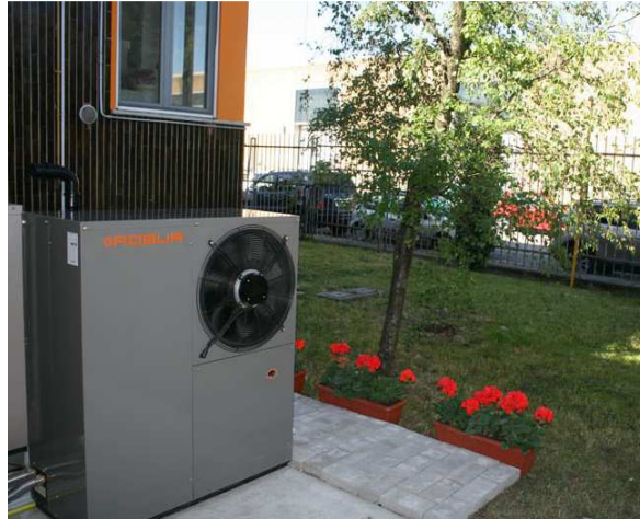
Figure 2: Example of installation of a residential GAHP in an existing building
