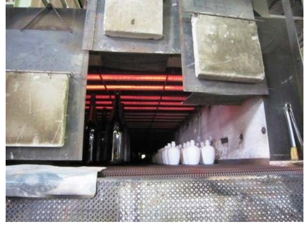
Fig3 Entrance of the annealing furnace
