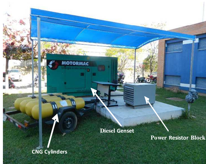
Figure 2 - Facilities operating tests of the Dual Fuel system
