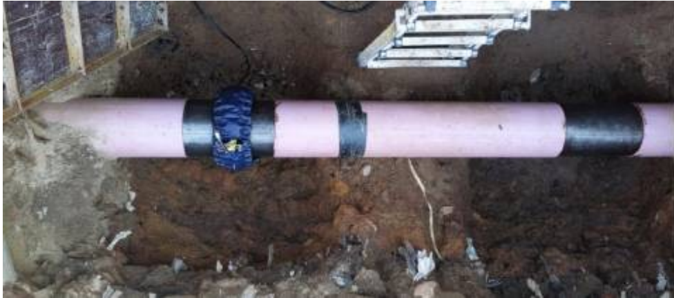
Figure 10. Inspection with piezoelectric sensor at valve station
