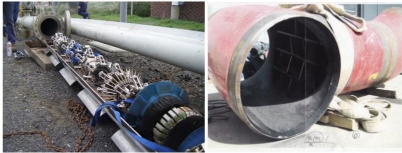
Fig. 8 pig and t-branch pipe with pig bars
