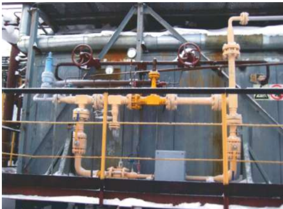
Fig.4 3S-separation unit at Zapolyaroye field of Gazprom
