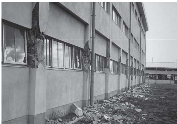
Photo1 Short RC Column's shear fracture by Tokachi-oki Earthquake in 1968 1)
