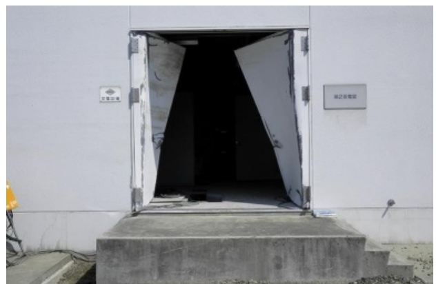
Photo 5.1 Transformer room's door was broken by the Tsunami
