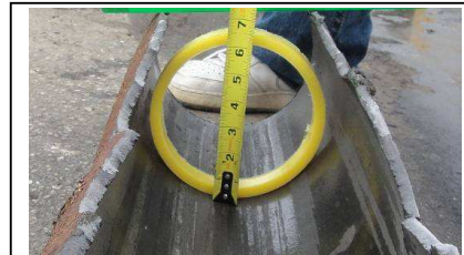
[Fig. 6] Cut open cast iron pipe and PE pipe
