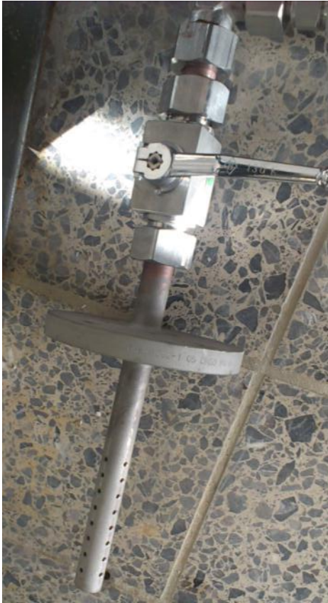
Lance for hydrogen injection
