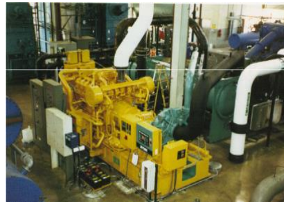
Gas Heat PUMPs
