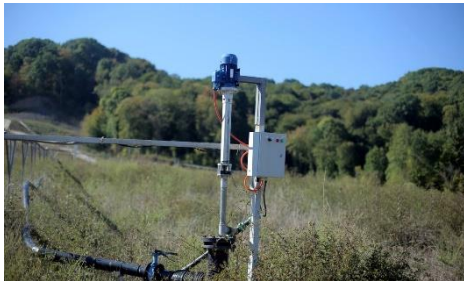
gas drainage well
