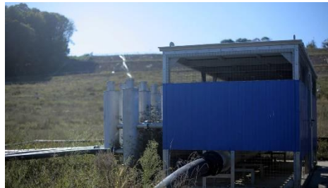
gas collection unit
