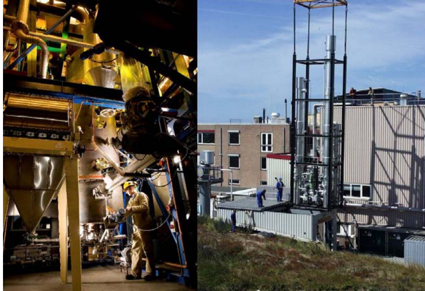
Figure 8: Pilot-scale MILENA gasifier (left) and installation of the OLGA pilot-scale gas cleaning (right).
