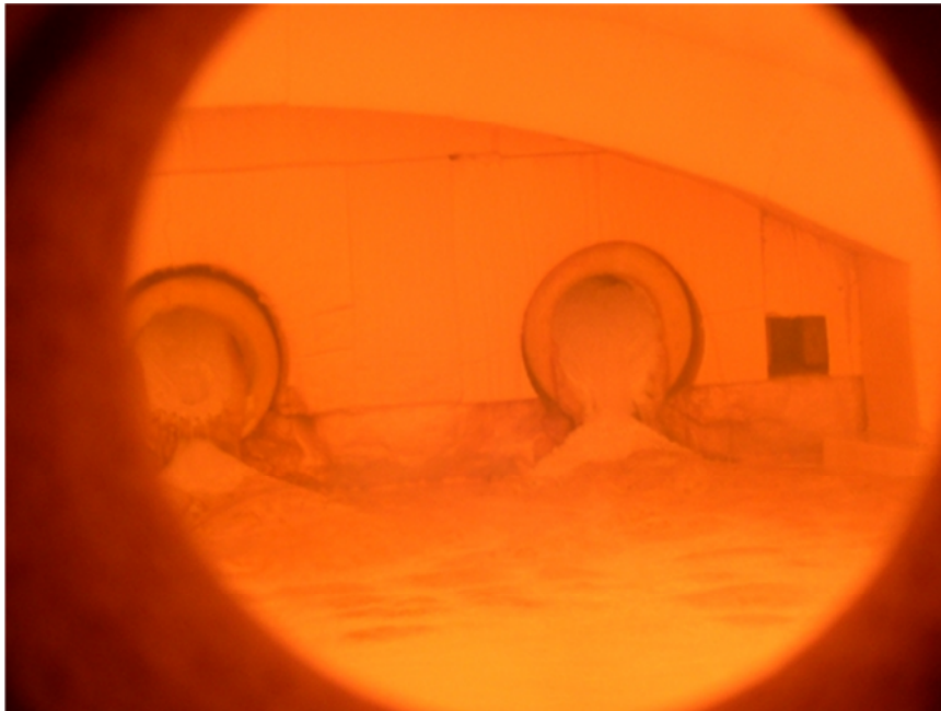
Figure 10: View into an operational GlasFLOX furnace
