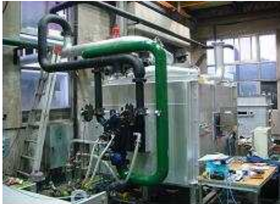
FIG. 1 Self-regenerative burner system in the test furnace
