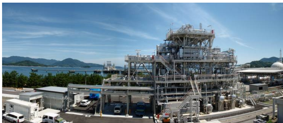
Figure 7: NGH production plant with 5 ton-per-day capacity built in Yanai LNG-based Power Station of CEP
