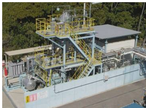
Figure 6: BSU plant in MES Chiba Works
