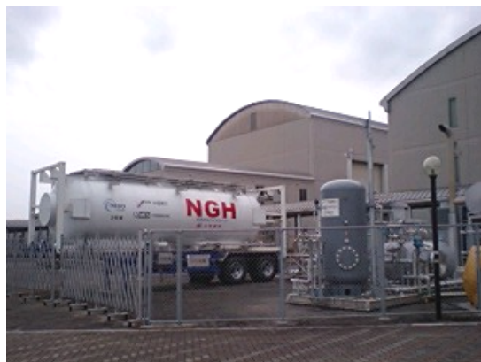
Figure 14: Gas Engine Power Generator Site (User 1)
