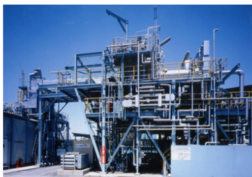
Figure 5: PDU plant in MES Chiba Works
