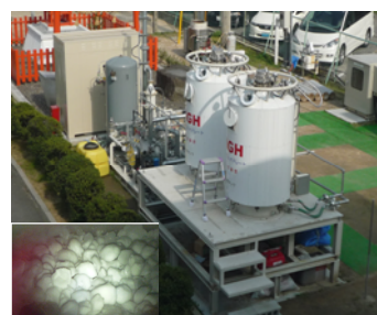
Figure 15: Testing facility equipped with home appliance (User 2)
