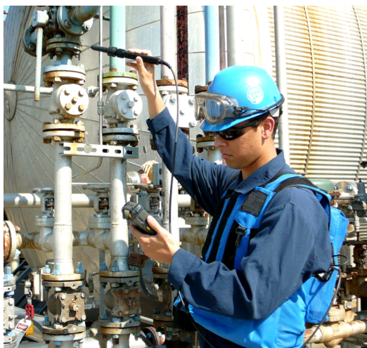
Figure 2 – Method 21 uses an organic vapor analyzer (OVA) or toxic vapor analyzer (TVA). The component is approached and, “sniffed,” to record the leak concentration. Here the gasket seal of valve flange is monitored. Photo courtesy of Team Industrial Services
