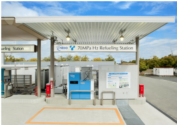
Photo. 2 Appearance of the 70 MPa hydrogen refueling station in Toho Gas Technical Research Institute
