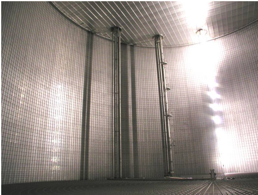
Figure 5: Internal view of a membrane containment tank
