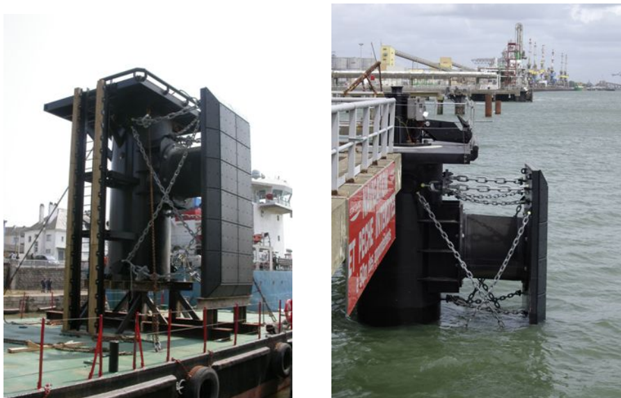
Figure 25: For each pile, a prefabricated fender module pile head is installed and commissioned
