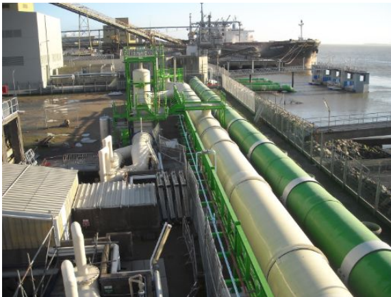
Figure 30: Synergy water pipes (from terminal)
