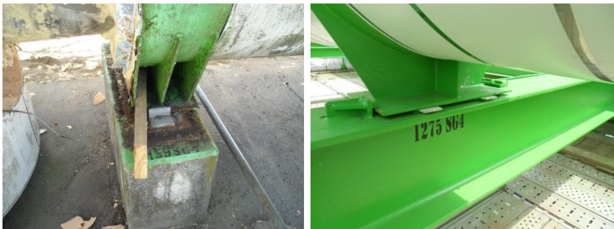
Figure 7: Corrosion impact on a pipeline support system (before and after replacement)
