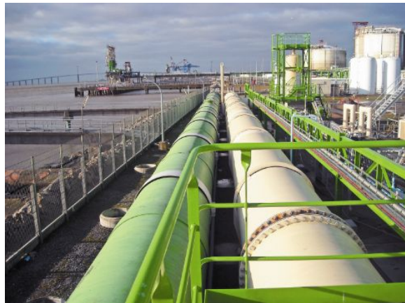
Figure 31: Synergy water pipes (from power plant)
