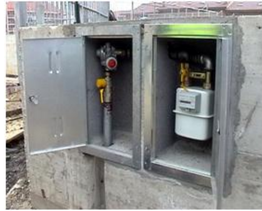
Figure 4.19 Gas Meter (Usually a diaphragm meter for home use)
