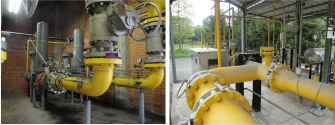
Figure 4.17 City gate: Plant for receiving, reducing and measuring gas provided by a transmission pipeline
