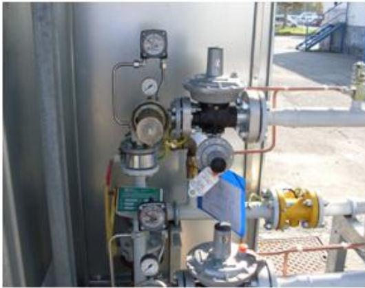
Figure 4.18 Medium pressure reduction plant
