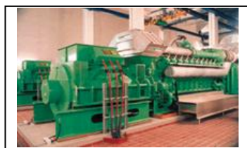
1000kW Biogas engine
