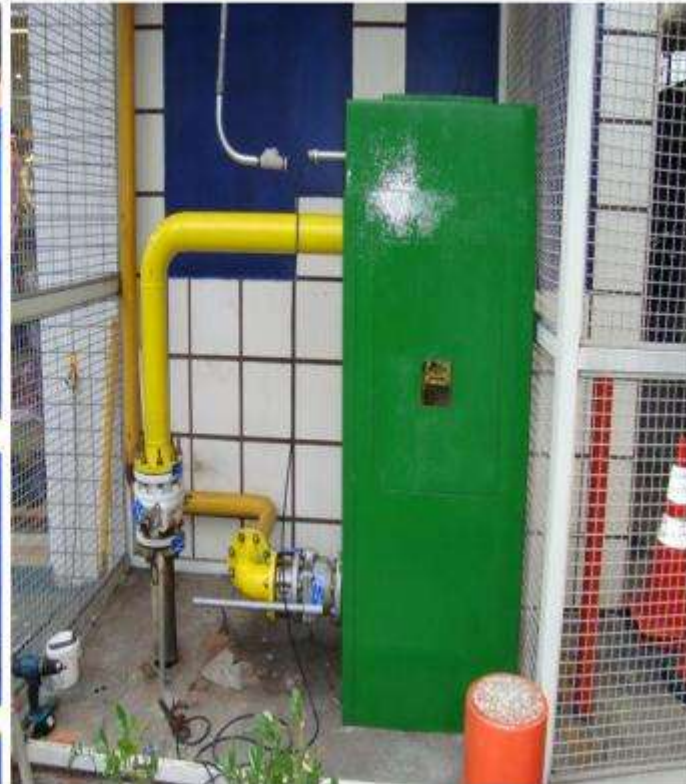
NGV Station A: after (meter with PU and with the box)
