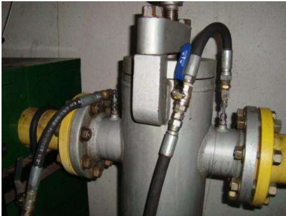
By Pass at Filter Pressure Gauges
