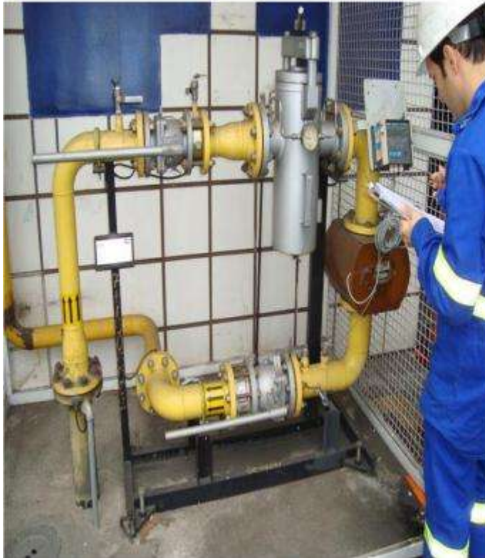
NGV Station A: before (meter with PU, without the box)
