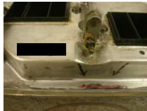
Figure 13 – Leakage from the internal case of an animal diaphragm meter
