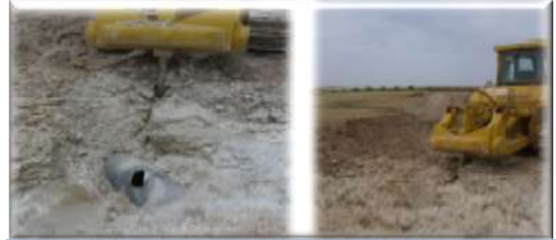
Works of opening of trench for the pose (installation) of the pipe Medgaz (Chentouf W Temouchent (Cosider-Sonatrach, Algeria) damaging a pipe of gas-- emergency intervention.
