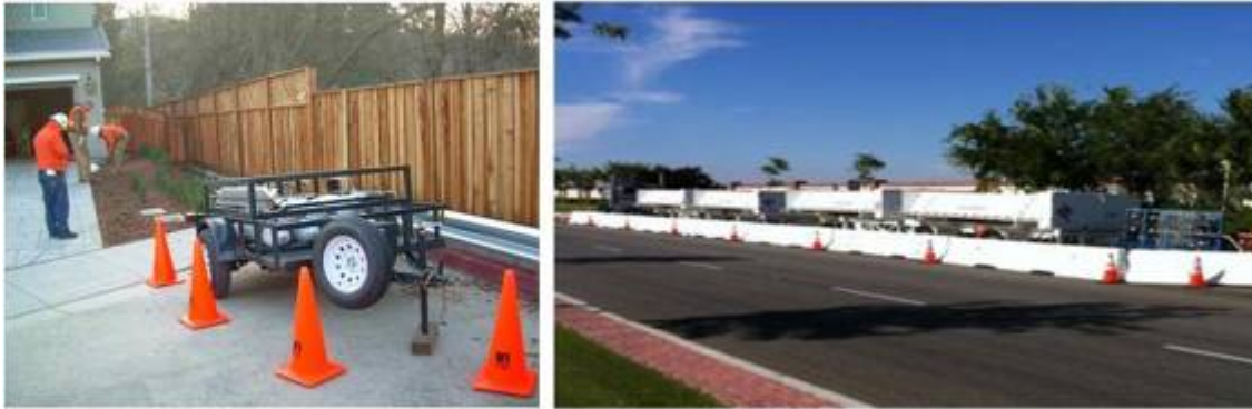
Figure 29. Equipment PG&E uses to preserve service during hydrostatic testing
