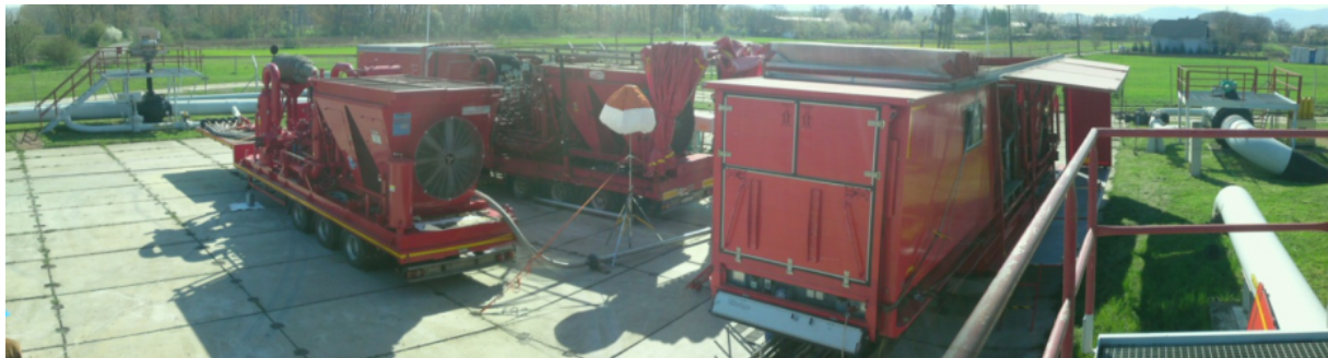
Fig. No.1. The use of three mobile compressors for gas re-pumping.
