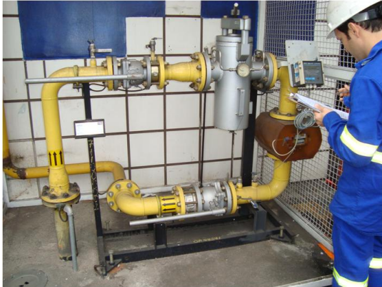
NGV Station A: before (meter with PU, without the box)
