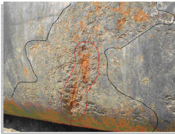
Corrosion: joint of spiral weld
