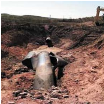
(Algeria), pipeline Hassi-R'mel-Arzew Mohammadia, corrosion - flight of gas explosion-fire, 78 persons hurt, damage to property - similar to a previous accident le19 in August, 2004
