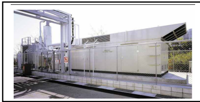
Picture 1 Biogas engine
