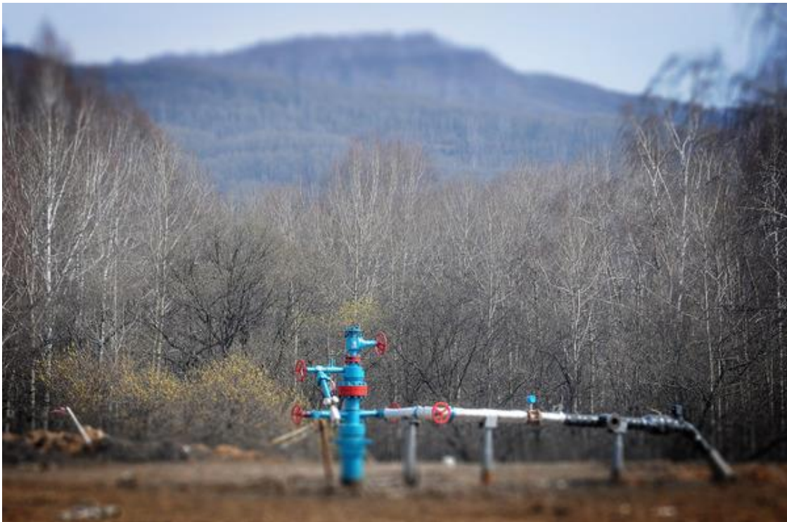
Fig. 4. Wellhead of horizontal coal-bed-methane well RN-11g with gathering line attached – the first well of such type in Russia
