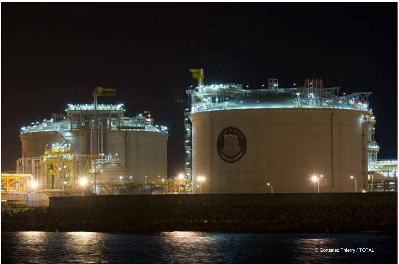
Storage Tanks at Yemen LNG, Balhaf, Yemen
