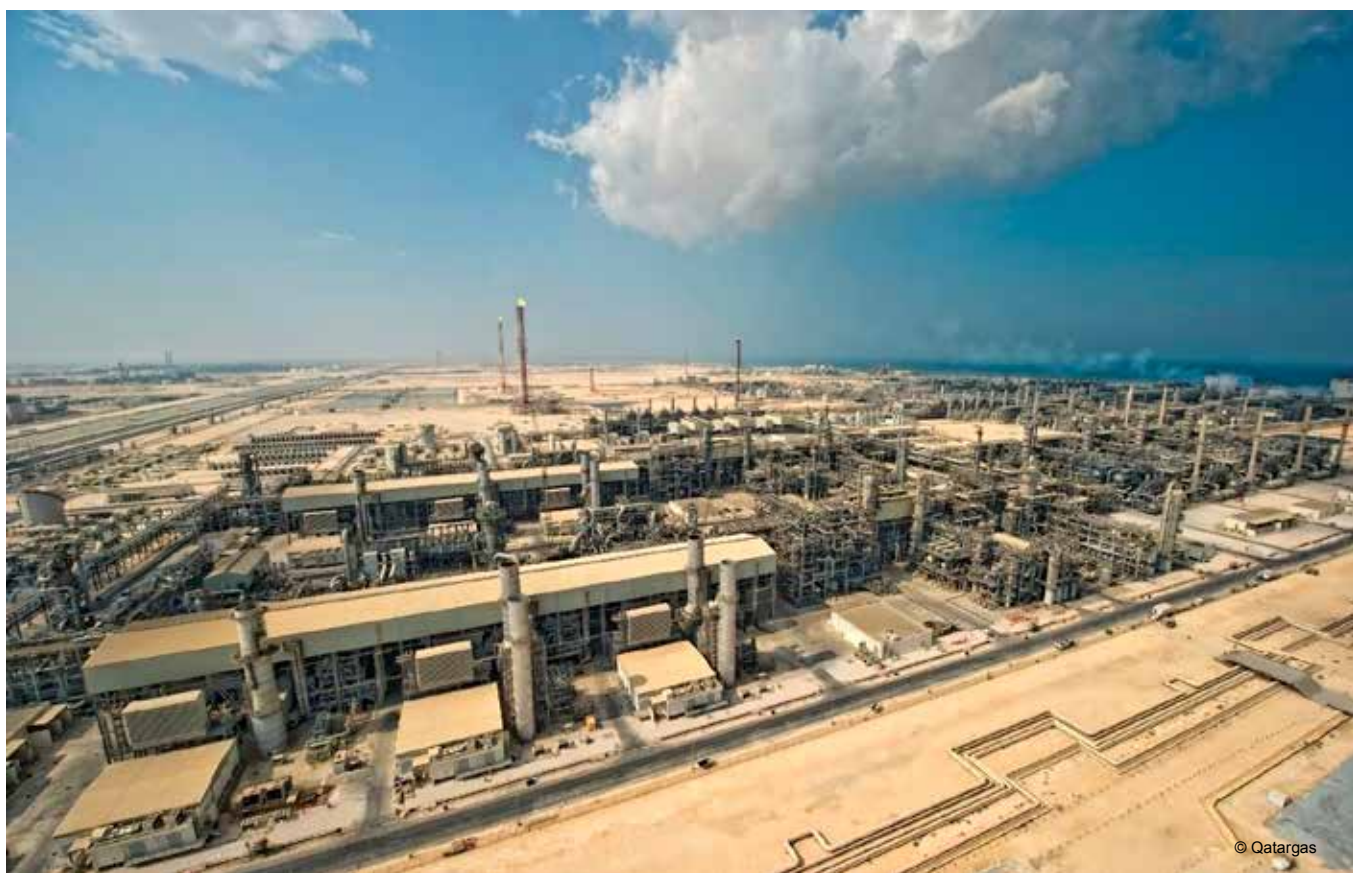
Qatargas Train 6, Ras Laffan, Qatar
